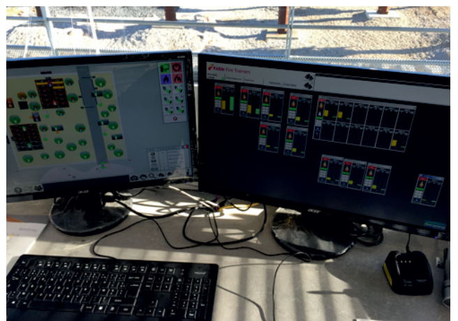
PC Control System
